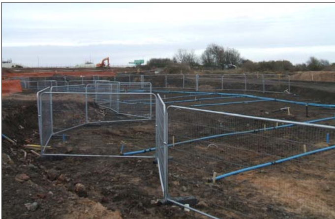
ABOVE GROUND PIPEWORK FOR SPARGE AND VAPOUR EXTRACTION
