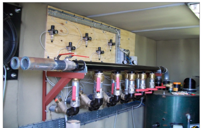
SOIL VAPOUR EXTRACTION MANIFOLDS
