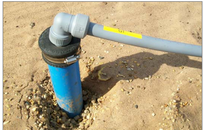
SOIL VAPOUR EXTRACTION WELL
