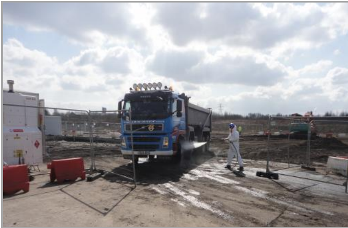
JET WASHING THE WAGONS EXITING THE CONTROL ZONE, PRIOR TO USING THE WHEEL WASH
