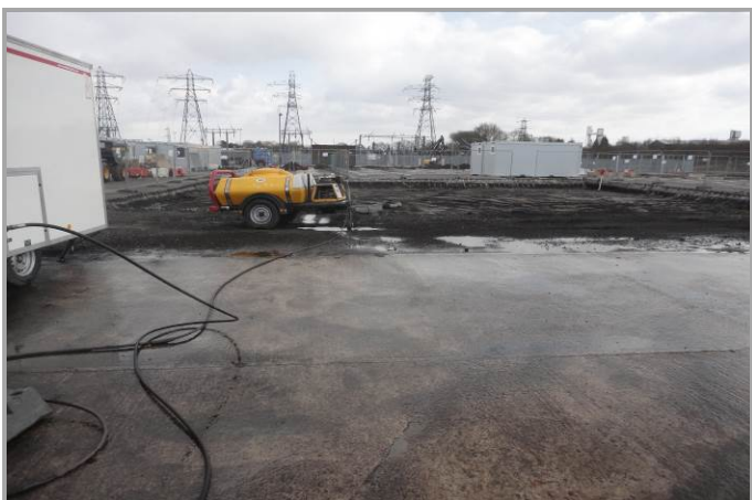
ACCESS AND EGRESS AREA OF A CONTROL ZONE SHOWING DECONTAMINATION UNIT AND JETWASH BOWSER
