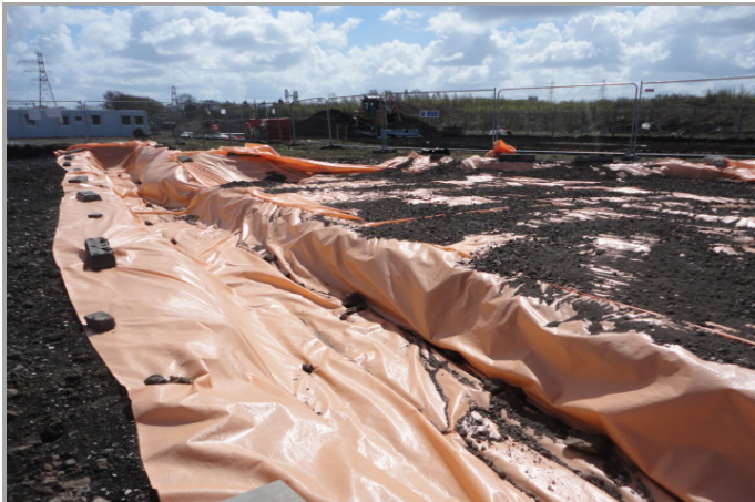
INSTALLATION OF WARNING GEOTEXTILE LINING ALL EXCAVATED SERVICE TRENCHES AND EXPOSED SITE AREA
